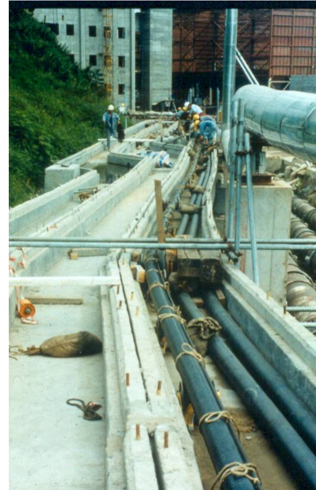
500kV Cables in China
