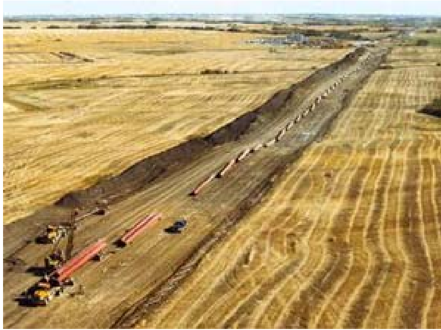
Figure 8-2 Example of gas pipeline being delivered to site in preparation for welding
