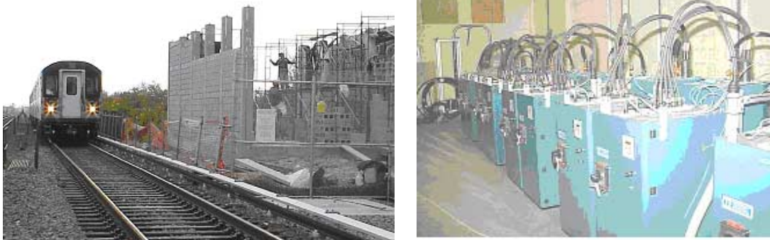
Figure 13-14 Flywheel Installation at NYCT Bay Equalizer Location, 10 100-kW Units in New Building
