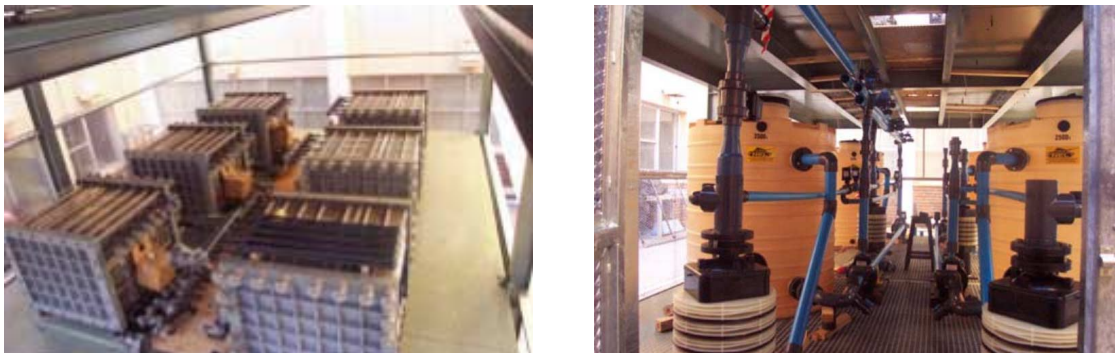
Figure 10-4 Typical VRB Stacks and Tanks (Courtesy VRB Power)
