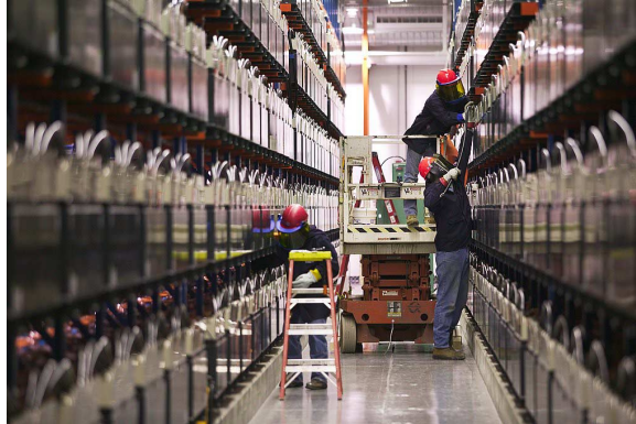
Figure 7-5 GVEA BESS NiCd Battery (Courtesy GVEA)
