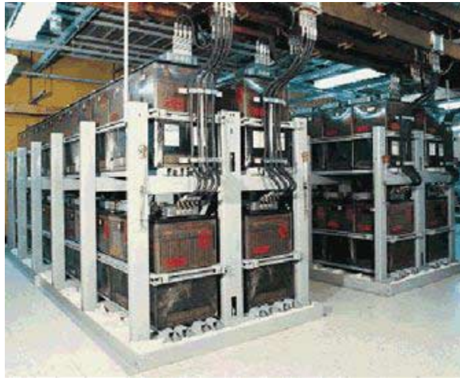
Figure 6-9 Stationary Battery Installation (Courtesy C&D Technologies)
