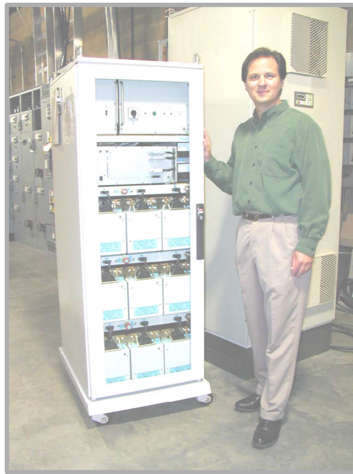
Figure 14-15 Electrochemical Capacitor System for DC Ridethrough
