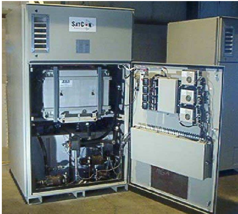
Figure 9-5 ZBB 50 kWh System With Integrated PCS (Courtesy ZBB Energy Corporation)
