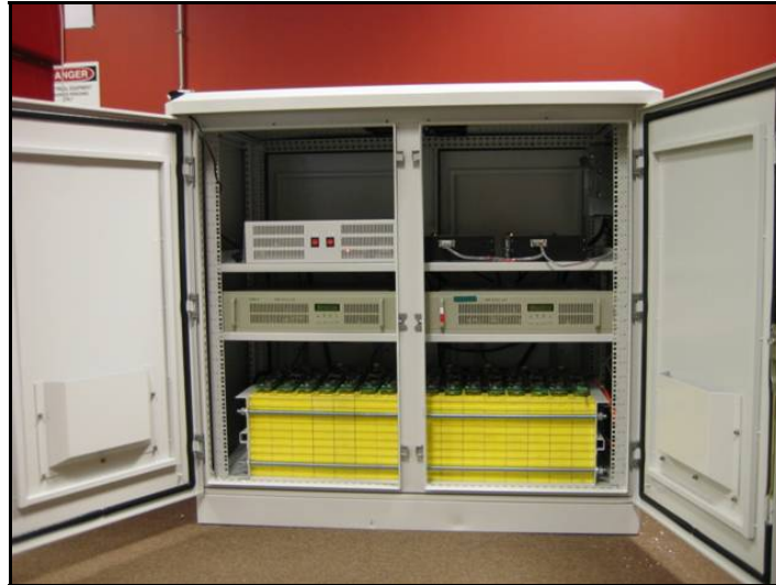
Figure 4-20 6-kW/20-kWh Li-ion system with inverter and controls by GreenSmith Energy Management. EPRI will be testing a 25-kW/50-kWh GreenSmith system in late 2010.
