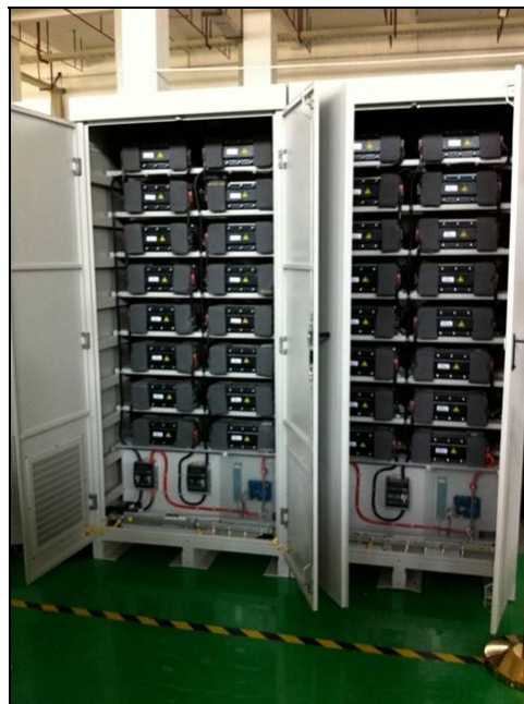
Figure 4-21 A 50-kWh BYD Li-ion Battery System Planned to be Tested at EPRI's Knoxville, Tennessee Smart Grid Laboratory in 2011.
