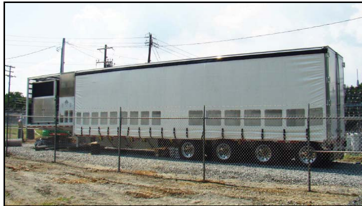
Figure 4 Premium Power's 0.5-MW/2.8 MWh TransFlow 2000 Transportable Zinc-Bromine Energy Storage System Preparing for Demonstration by EPRI.
