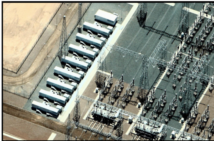
Figure 7 Commercial operation of a 12-MW frequency regulation and spinning reserve project at AES Gener's Los Andes substation in the Atacama Desert, Chile. The system uses A123 Systems' Li-ion Hybrid Ancillary Power Units (Hybrid-APUs™).
