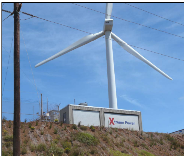
Figure 4-9 1.5-MW/1-MWh Advanced Lead Acid “Dry Cell” Systems by Xtreme Power being deployed in a wind farm application (Source: Xtreme Power).
