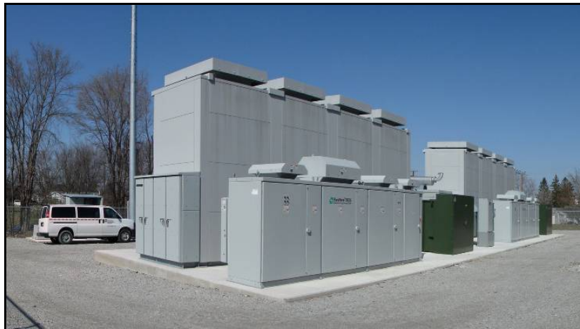
Figure 4-11 AEP Distribution Substation with Sodium-Sulfur Unit
