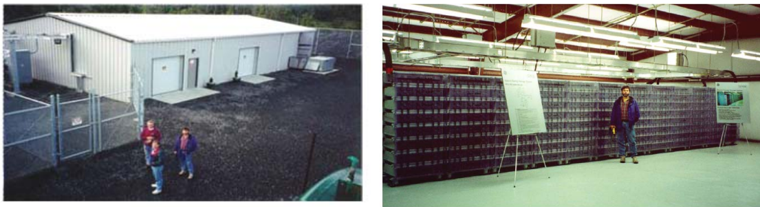
Figure 4-7 1-MW/1.5-MWh Lead-Acid System at Metlakalta, Alaska
