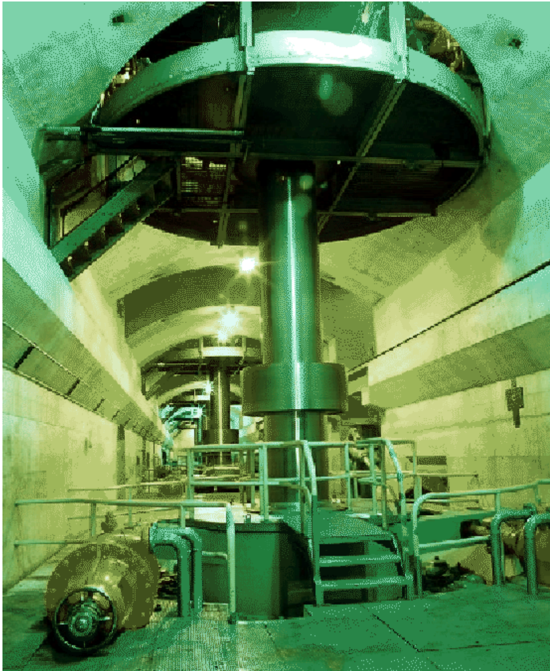
Figure 5.4: Inside of a generator.
