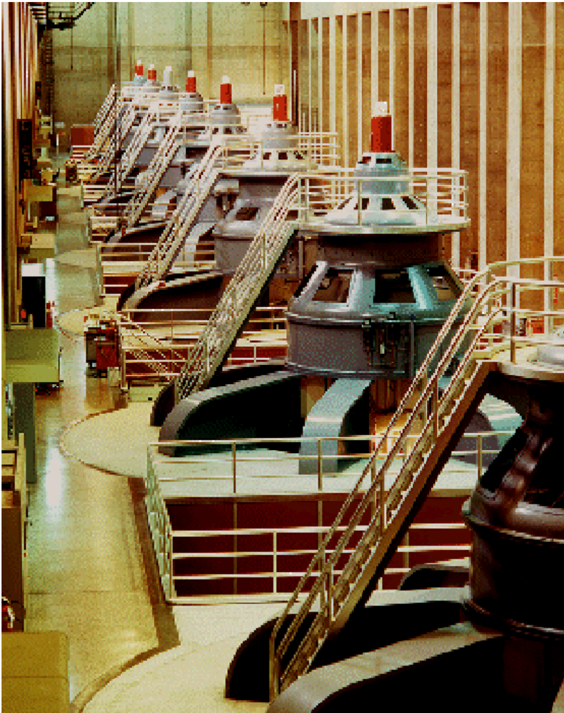
Figure 5.3: A series of generators.
