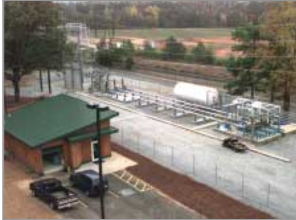
First use of HTS cables in an industrial application
